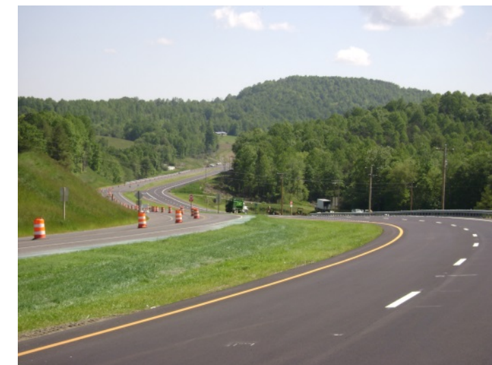
Laurel Fork involved widening and new roadway alignment through hilly terrain while maintaining access to 120 driveways and improving intersections with 14 secondary roads.
