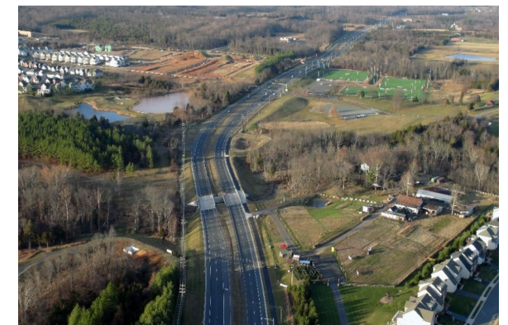
Route 15 construction required special attention to MOT to maintain safety of the traveling public and our work crews.
