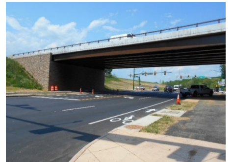
The Rt. 7/Battlefield Parkway has similar issues with an undersized culvert under Battlefield Parkway at Russell Branch Rd. SE.
