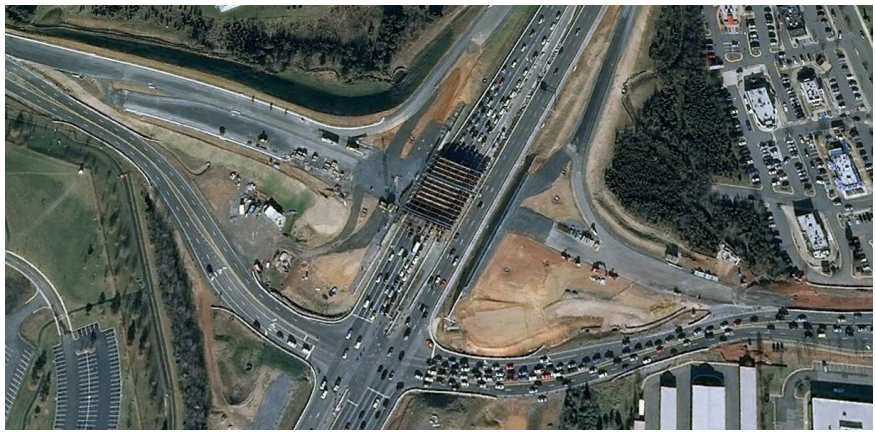
Figure 3.5.2 - Willard Road Diversion at Route 28 where all movements were maintained with a signalized intersection on a temporary alignment adjacent to bridge and ramp construction.
