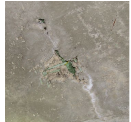
Figure 8: Inadequate Concrete Consolidation in the Longitudinal Joint Region
