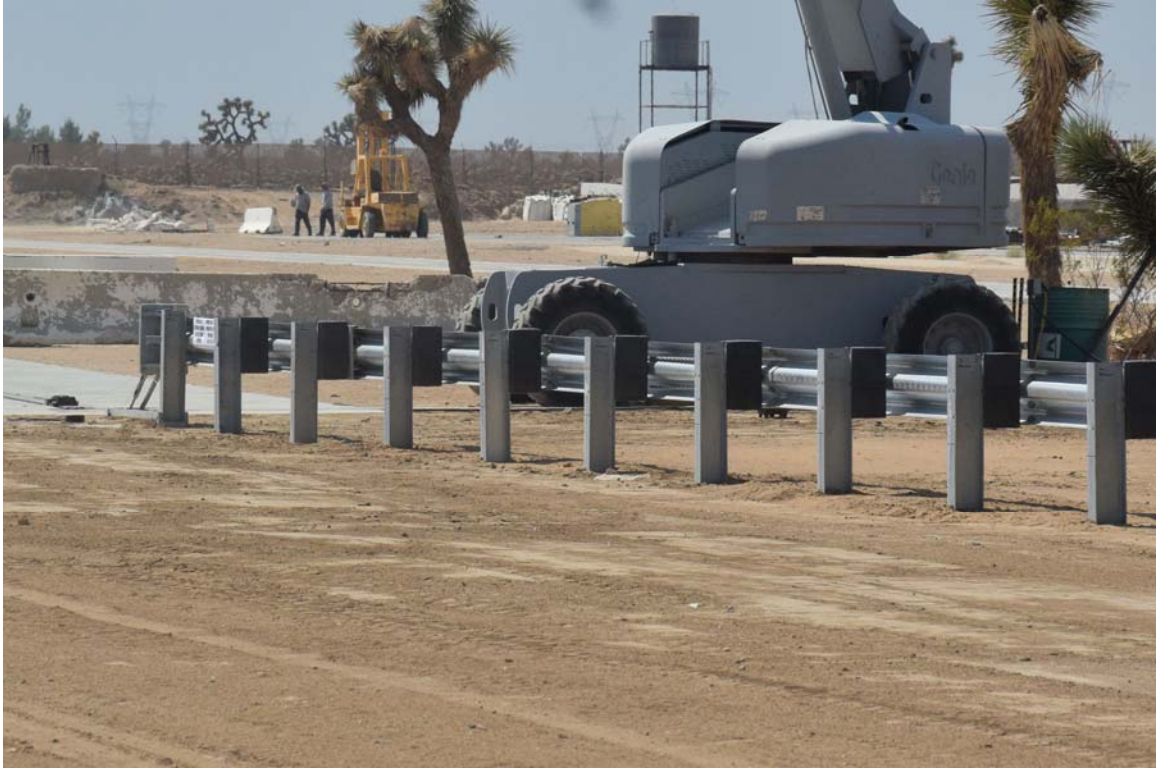
FIGURE 29. Pre-Test Left Rear \frac{3}{4} View of Test Article
