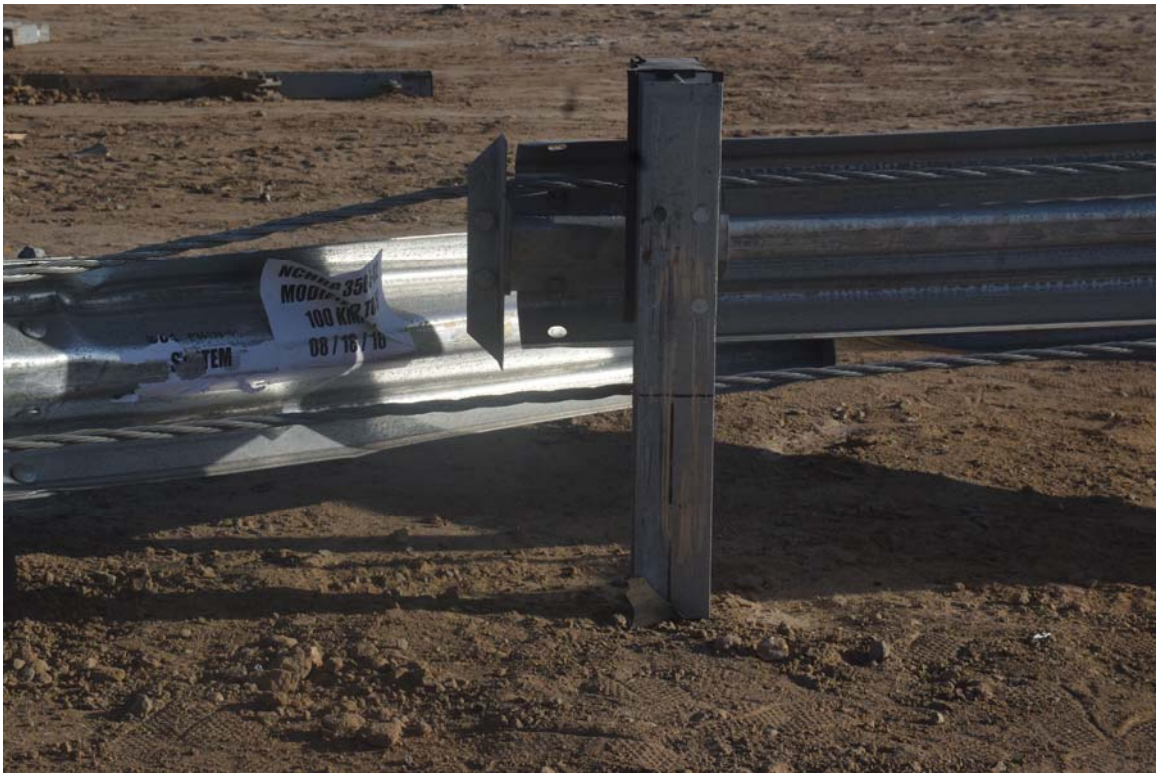
FIGURE 35. Test Article Damage
